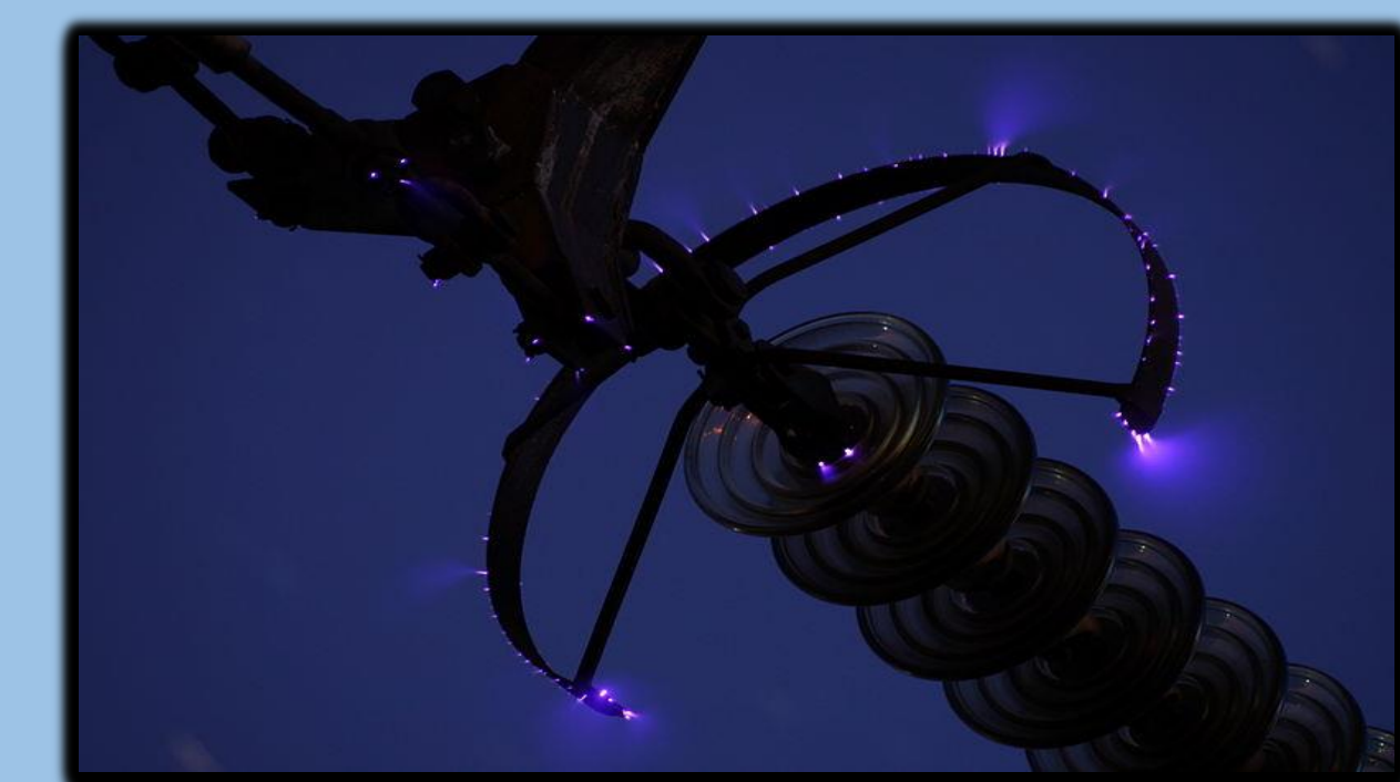
Figure 1: Glow Coronas form on the edges of a powerline transformer (Berkoff, 2005).
