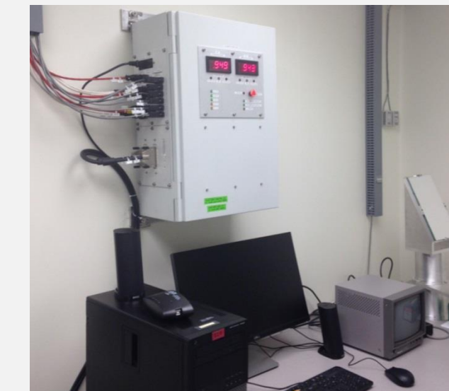
INSPIRe Control Room (Siderostat Control System, above)
